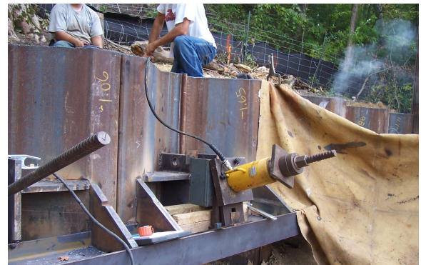
Proof loading of anchors to 133% design and locked off at 100% design load
