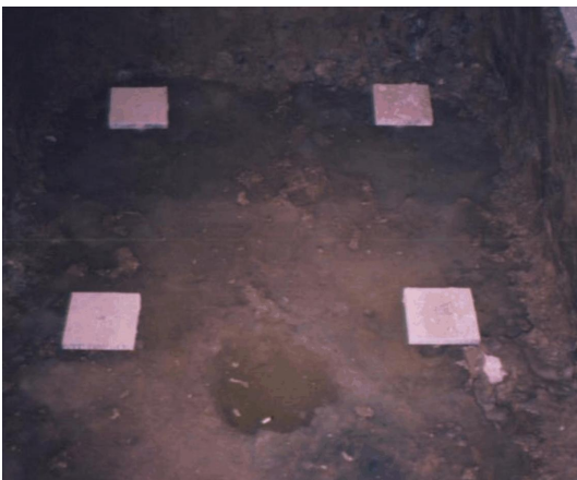
New construction brackets to be cast into new pile cap for elevator
